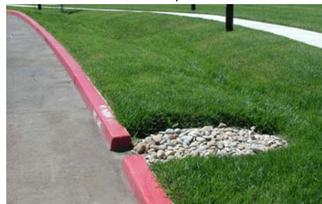
Figure 3-4: Cobbles help prevent erosion as stormwater enters treatment measure at Legacy Tech Park in San Jose. (Photo credit: RBF Consulting)
