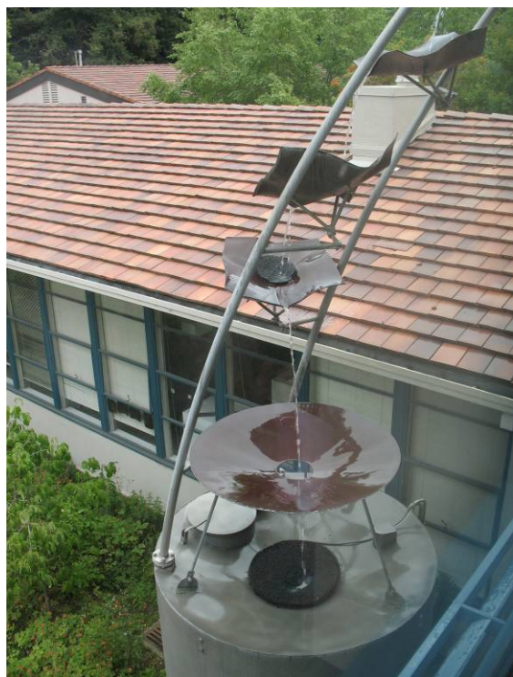
Figure 6-43: Rainwater is collected and used for flushing toilets at Mills College, Oakland.
