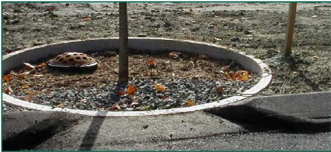
Figure 6-15: Non-proprietary Tree Filter with Overflow Bypass. Source: University of New Hampshire Environmental Research Group, 2006
