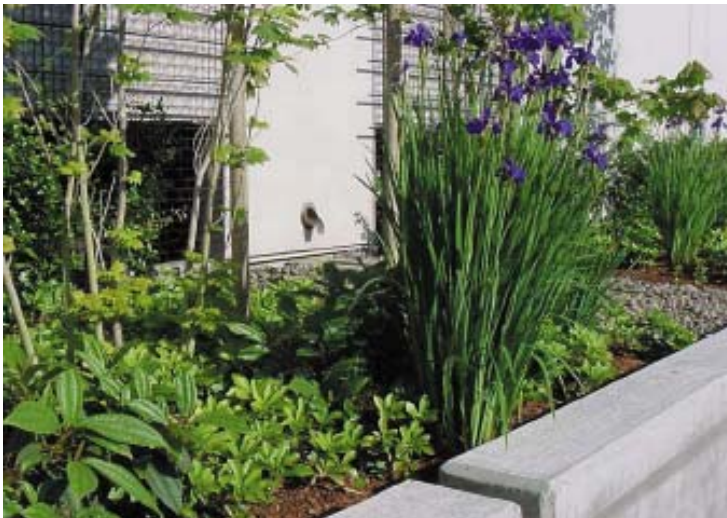
Figure 6-23: Close-up of Flow Through Planter. (Source: City of Portland)
