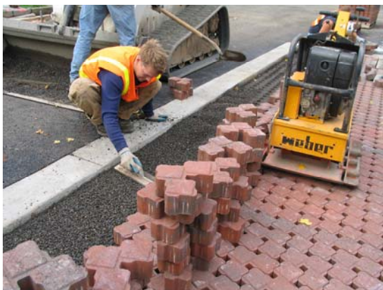
Figure 4-8: Installation of notched unit pavers in Portland, Oregon. Water infiltrates through notches between pavers. (Photo courtesy of City of Portland)
