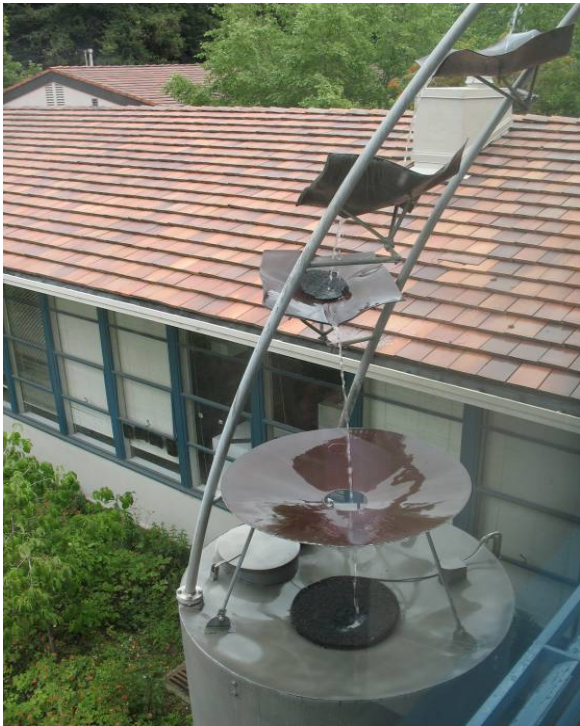
Figure 6-40: Rainwater is collected and used for flushing toilets at Mills College, Oakland.
