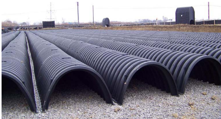
Figure 6-44: Photo of subsurface retention/infiltration system installation under a parking lot. Source: Contech.
