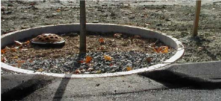
Figure 8-3: Non-proprietary tree well filter (Source: University of New Hampshire)
