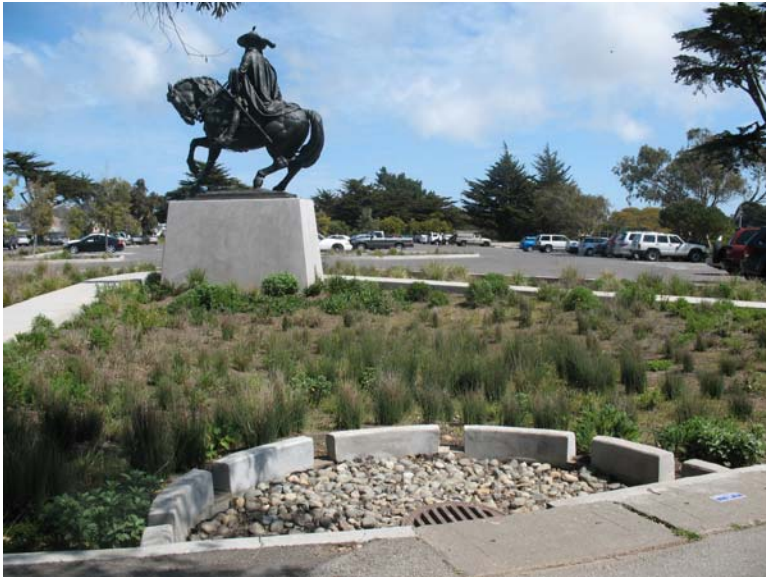
Infiltration Basin at Sunset Circle Parking Lot
