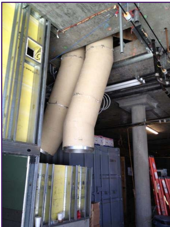
Figure 21. Problems during construction.
