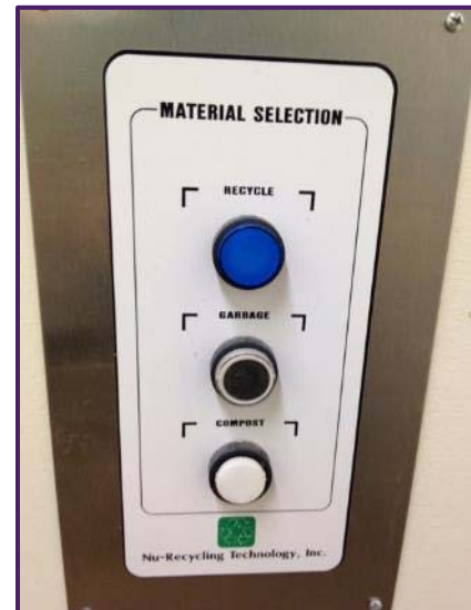
Figure 20. Button controls in chute room
