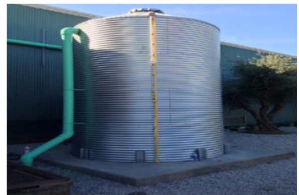
Figure 1-10 Rainwater harvesting cistern, Environmental Innovation Center, San José
