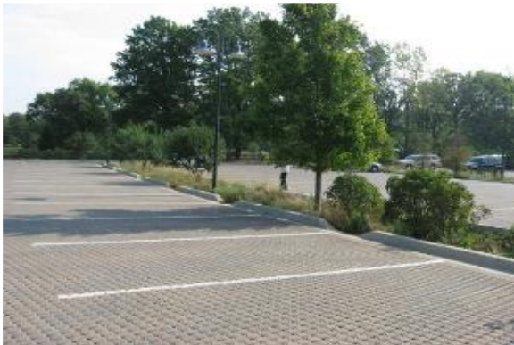
Example 2: LID (Pervious paving in a parking lot)
