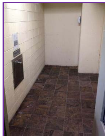
Figure 13. Chute room with one garbage chute door and no recycling or composting options
