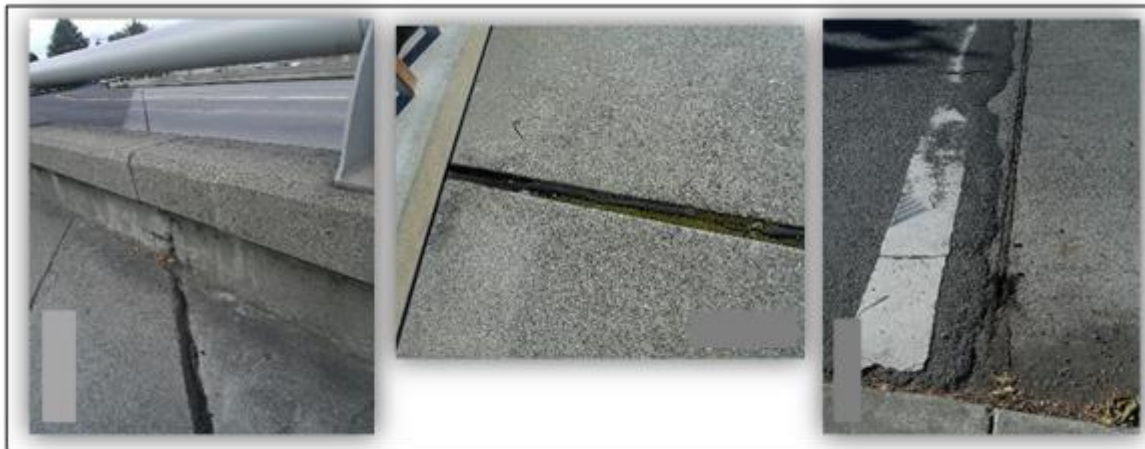
Figure 3.6 Examples of structures that were sampled and caulk materials that were included in Composite B, which had Very High PCBs ( \geq 1,000 ppm).
