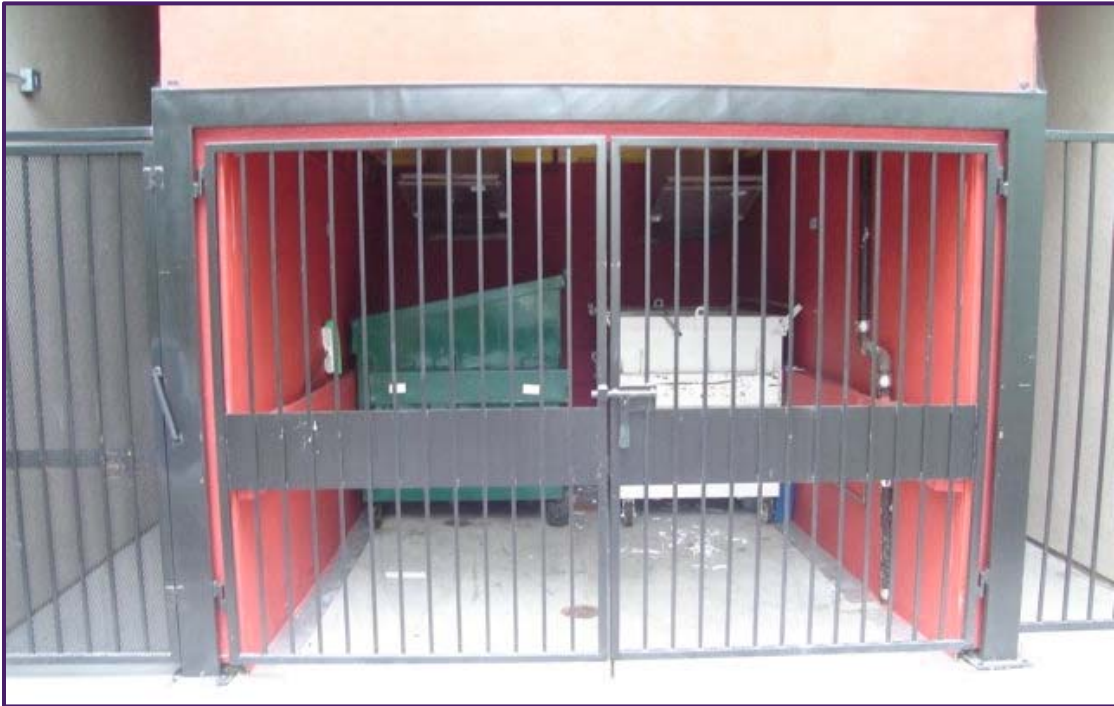
Figure 16. Dual chute enclosure with access gates for hauler
