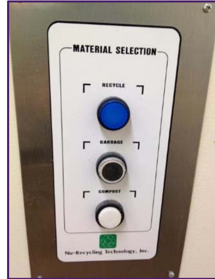
Figure 20. Button controls in chute room
