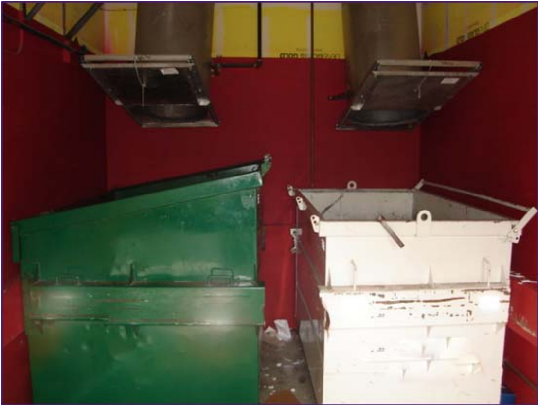
Figure 15. Chute Room with dual chutes for recycling and garbage
