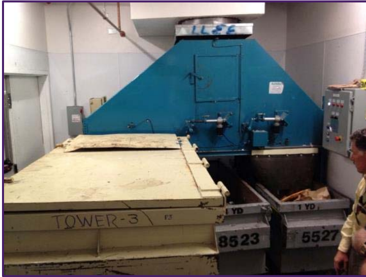
Figure 19. Tri-Sorter with compactor for garbage.
