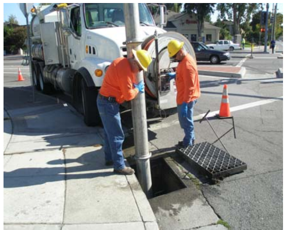
Figure 3-7. Operation and maintenance of an inlet-based trash control measure.
