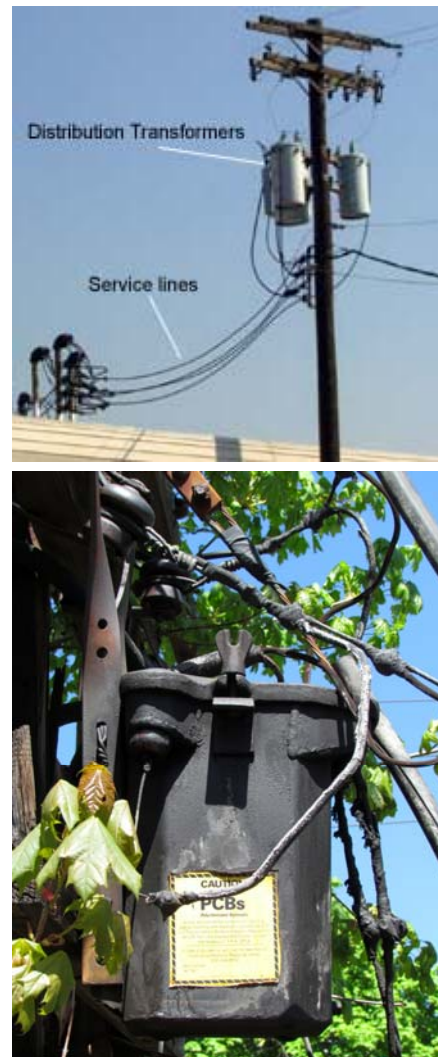
Figure 3-4. Pole-mounted electrical transformers with PCBs-containing oils.
