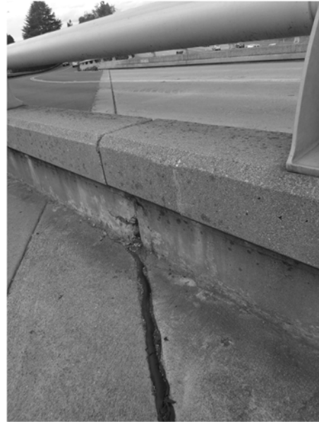
Figure 3-5. PCBs-containing black caulk materials on a roadway overpass structure.
