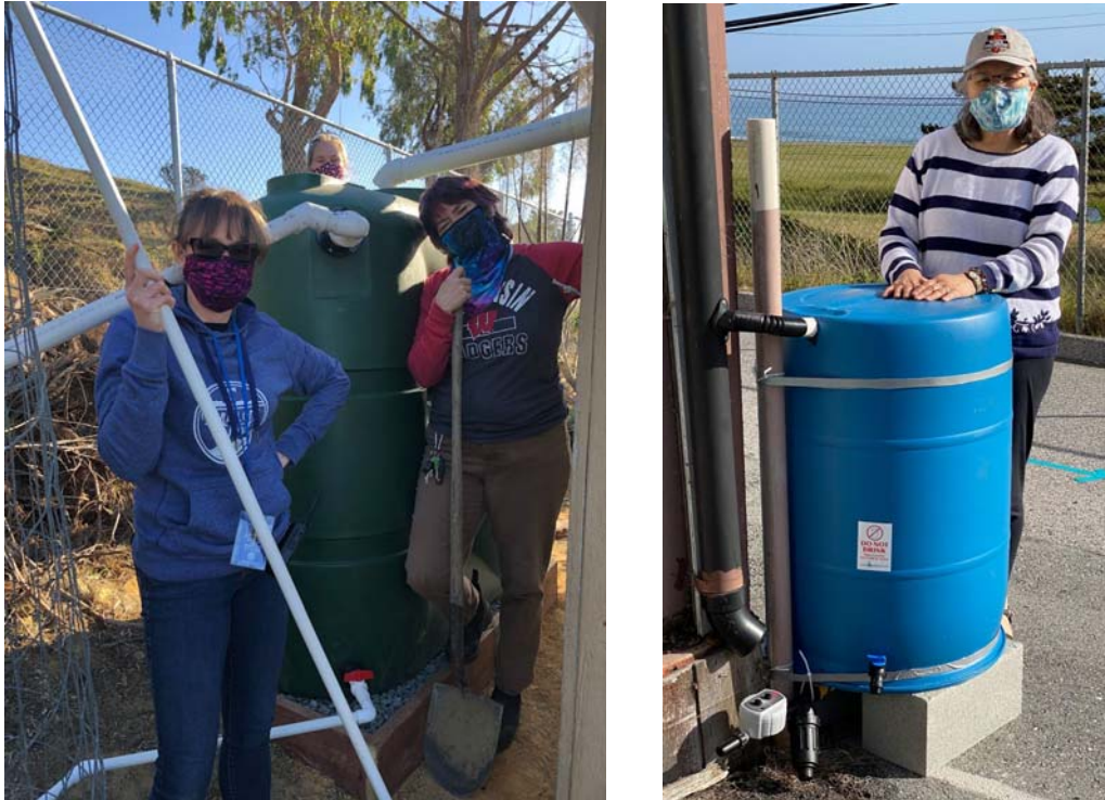
Figure 7-12. Photos of completed barrel installations at the Farallone Elementary campus (pictured left) and El Granada Elementary campus (pictured right)
