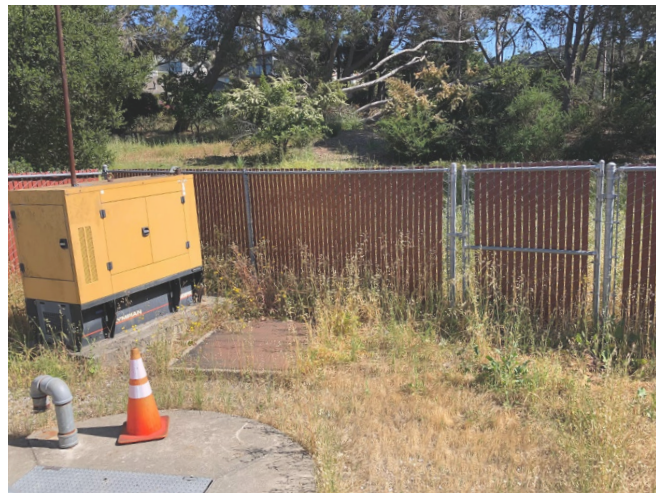
Septic infrastructure on site
