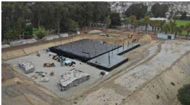
Regional facilities, which are GSI measures that treat runoff generated from a larger area, such as a neighborhood photo7
