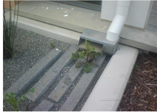
Figure 3-4: Splash block/box and flow spreaders help prevent erosion as stormwater enters treatment measure. (Credit: EOA, Inc.)
