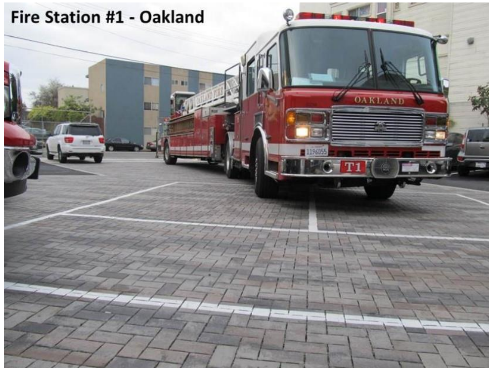
Figure 4-9: Installation of permeable interlocking concrete pavers in Oakland. Water infiltrates through gravel in the joints between the pavers. (Courtesy of the City of Oakland)
