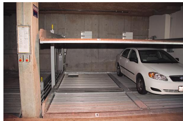
Figure 4-10: Parking Lifts in Parking Garage, Berkeley (Courtesy of City of Berkeley)
