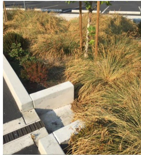
Figure 5-13: The side wings and concrete apron of this trench drain curb cut prevent blockage & erosion. (Credit EOA, Inc.)
