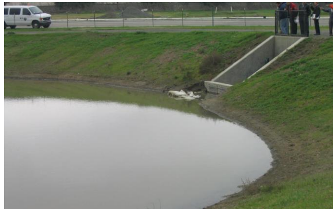
Figure 5-6: Detention pond used for hydromodification management.
