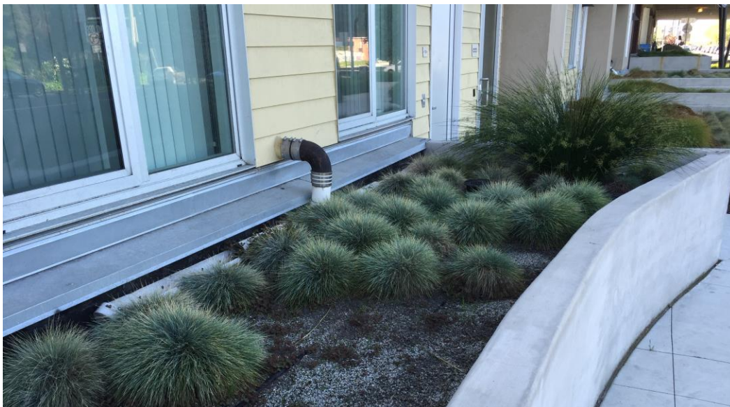
Figure 6-14: Close-up of flow-through planter with flow spreader. (Credit: EOA, Inc)
