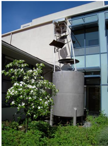
Figure 8-9: Rainwater Harvesting Cistern in Oakland at Mills College (Credit EOA, Inc.)
