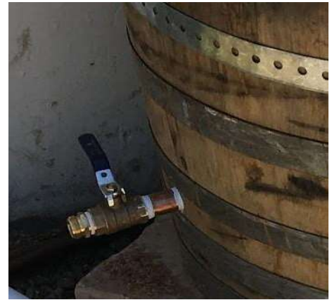
Figure 10: Outlet using ball valve
